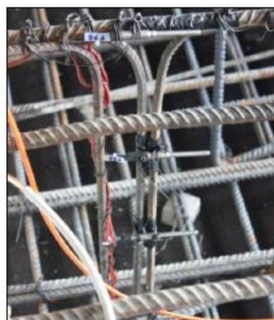
Figure 13 – Thermometers inside concrete
