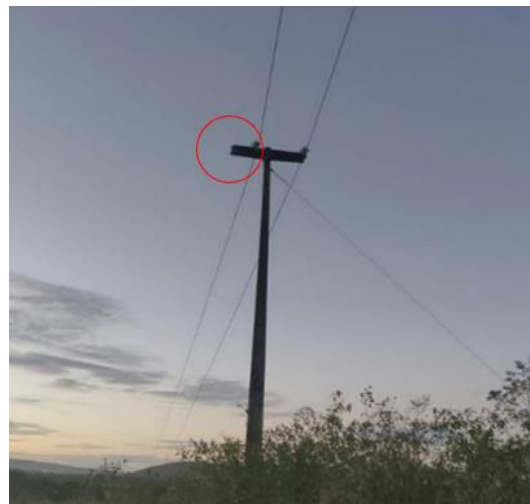
Figure 2 – Suspension structure with broken crossarm.
