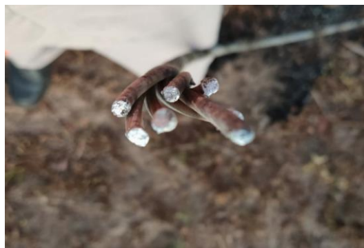
Figure 5 – Broken aluminum conductor wire.
