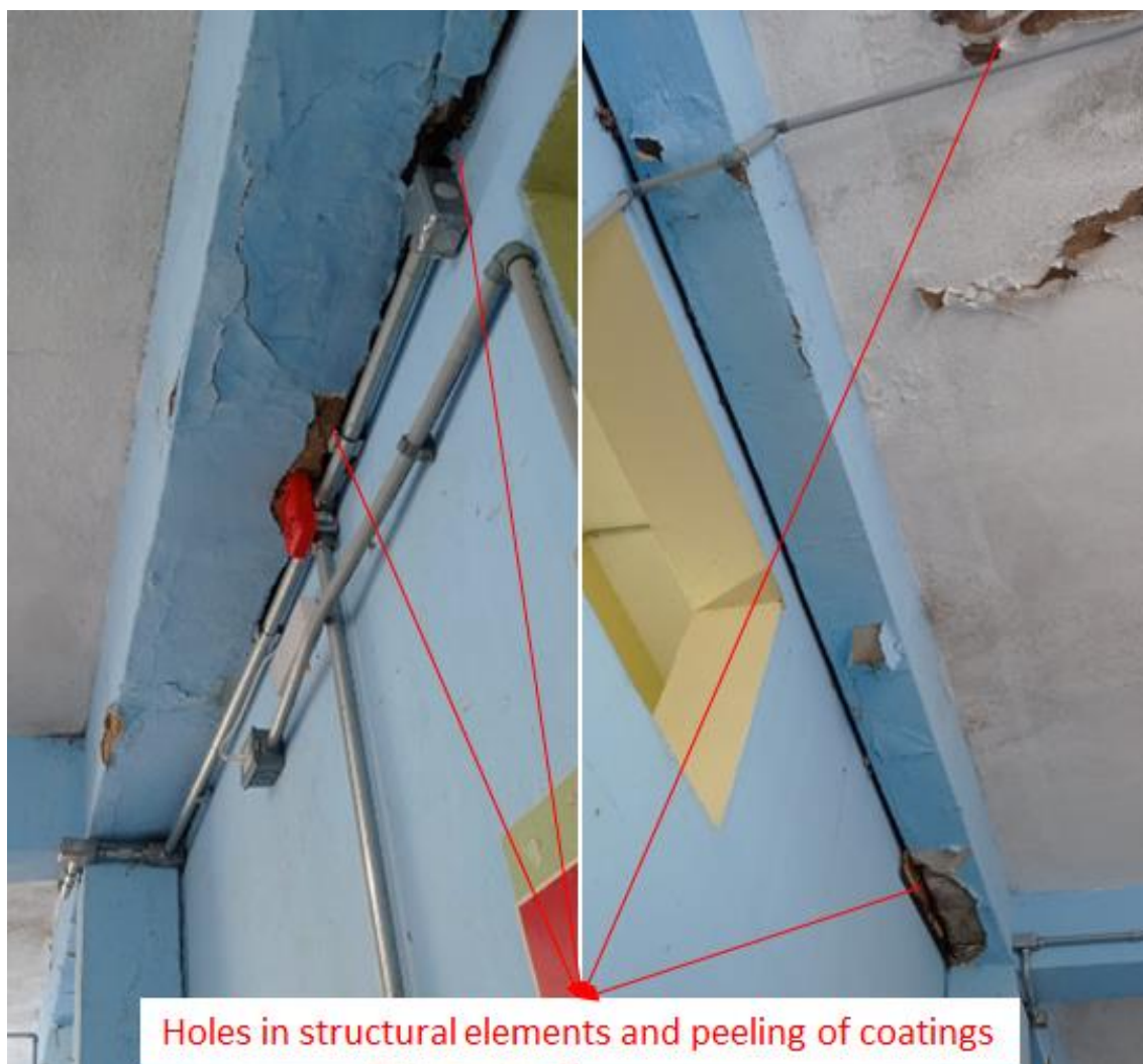
Figure 4 – Holes in reinforced concrete beams for passage of conduits. Source: Developed by the authors
