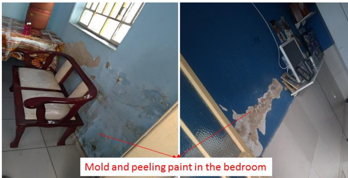
Figure 6 – Molds and peeling from soil moisture. Source: Developed by the authors
