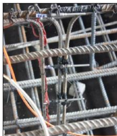
Figure 13 – Thermometers inside concrete
